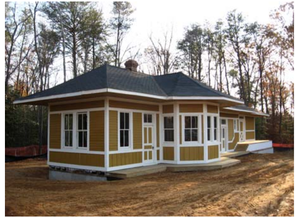
Depot Phase II Exterior Restoration complete. Fill dirt donated and site rough graded.
